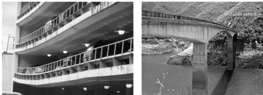
Fig. 1: Time-dependent deflections of RC slabs and beams at a Garage Parking in Pittsburg (left) and main post-tensioned girders of a bridge in Northern California (right) due to creep and shrinkage
